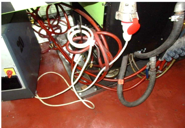
Figure 2 – Workplace with Implemented OHSMS Prior TPM Implementation according to IATF (Author's Elaboration)
